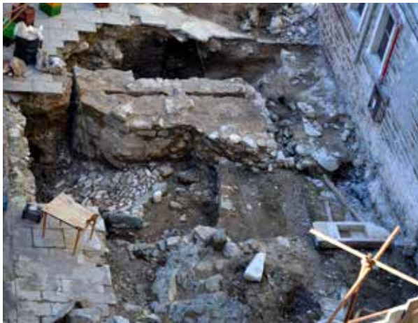
Fig. 8. St Paul's monastery; the revealed part of the Branković building and the part of the older stone-paved floor
