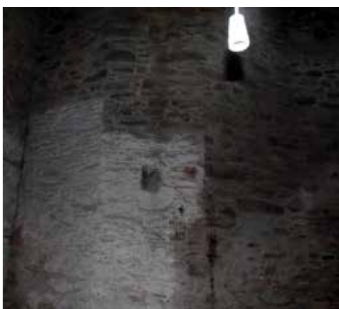
Fig. 12. Monastery of Philotheou; western wing; the structure with the refectory on the highest level; the northern wall with the apse
