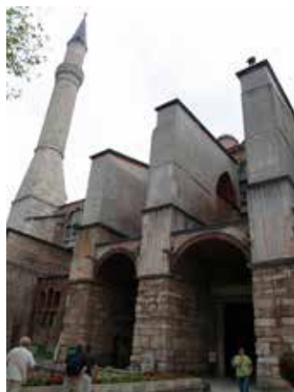
Fig. 7. Second and third buttresses of the west façade, Hagia Sophia in Constantinople, photo: Jasmina S. Ćirić
