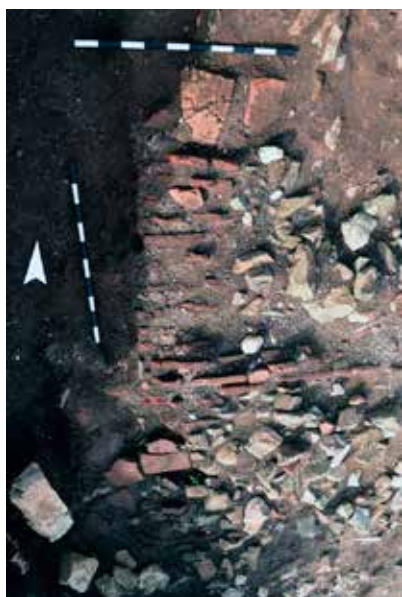
Fig. 2. The fallen from the earthquake northern wall of the basilica in opus mixtum .
