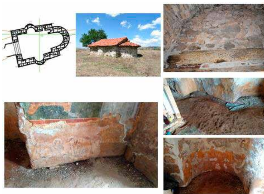
Fig. 12. The stylobate of the basilica: “foundations” of the medieval church. Wall painting over granite blocks – on the straight walls and in the northern conch.
