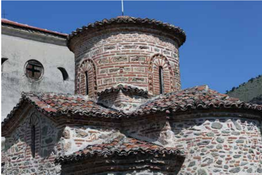
Fig. 10 Church of St Germanus at Prespa. The dome. Early 11 th century. Photo by the author.
