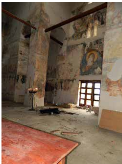
Fig.4. Interior of the Church of the Holy Mother in Mateič, visible damages, photo: Jasmina Zisovska
