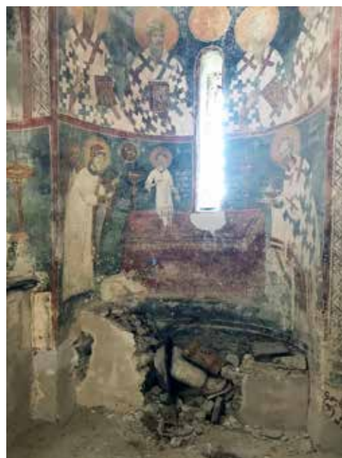
Fig.5. Damages inside of the apse, eastern part of the church, photo: Jasmina S. Ćirić
